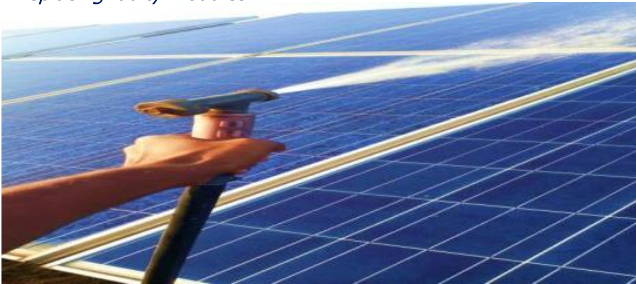
4 CYCLE CLEANING OF MODULES WITH MODULE CLEANING SYSTEM
